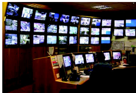
Figure 6: CCTV Control Room
